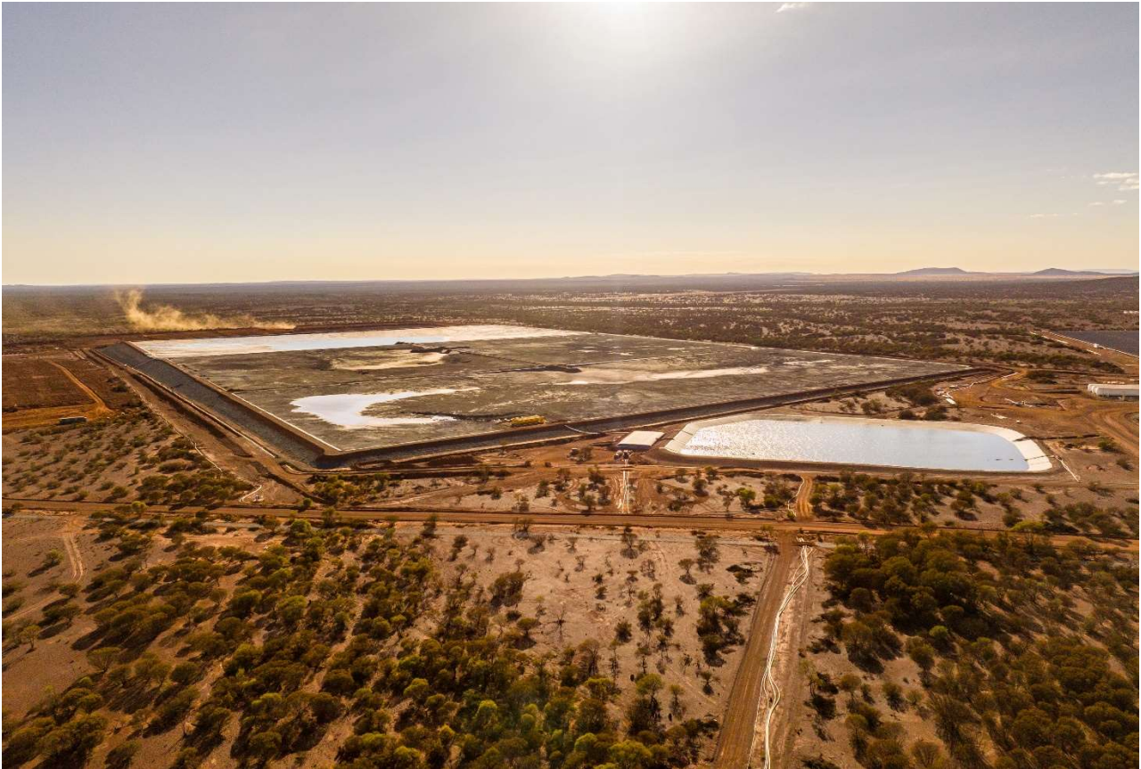
Figure 8 - TSF Cell A with earthworks on TSF Cell B2 ongoing in the horizon
