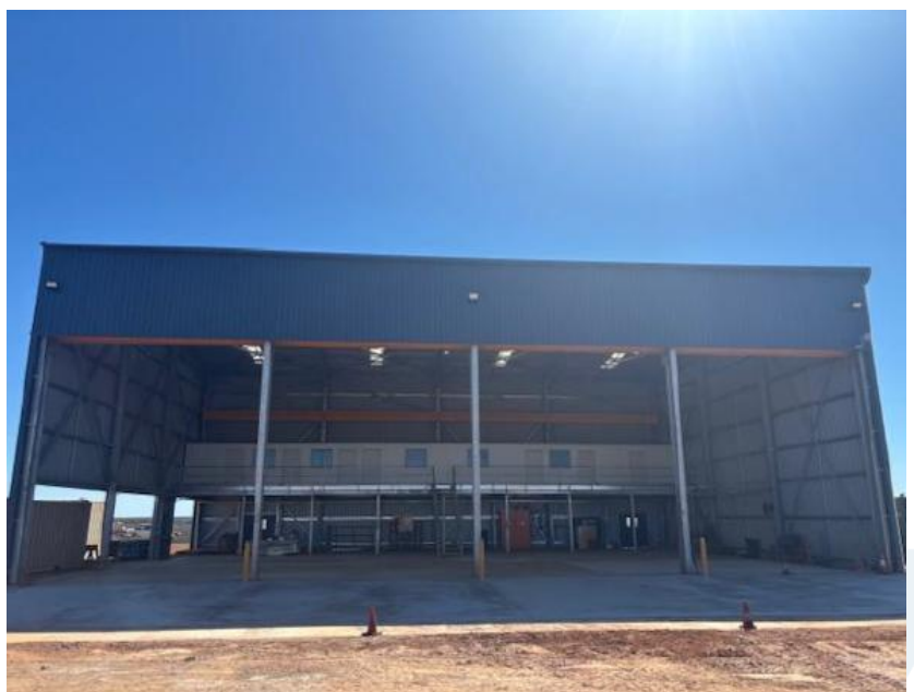
Figure 16 - Surface mobile maintenance workshop
